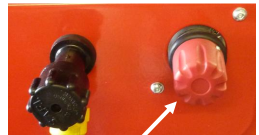
Battery Isolator Switch
