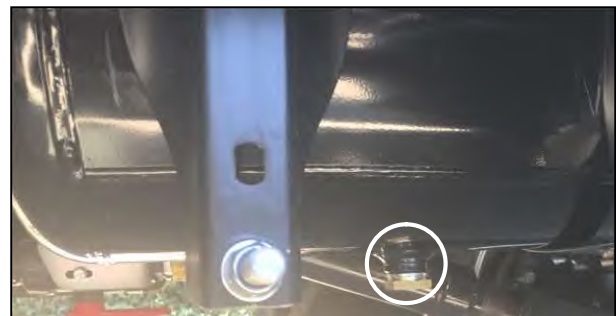
Air Tank Auto Drain Valve
