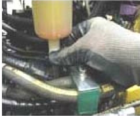
Water Drain Valve
