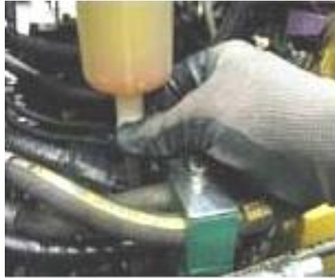
Water Drain Valve
