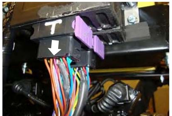
Disconnect the wiring loom plug from the Brake Control Module to allow machine operation with Manual Control
