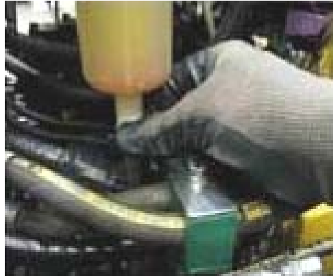
Water Drain Valve
