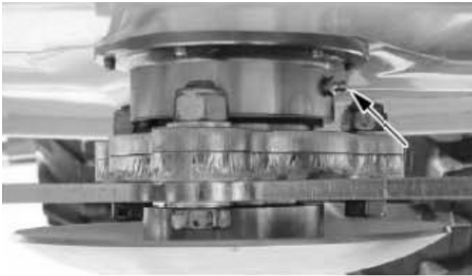
Bearing lubrication point
